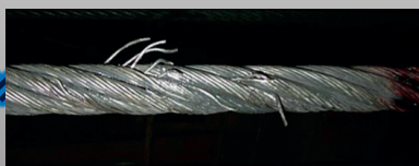
Wire break with protruding wire pieces
